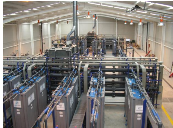
Figure 4: Installed EDR Systems
