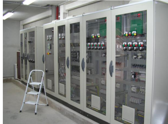
Figure 3: Controllers for the EDR System
