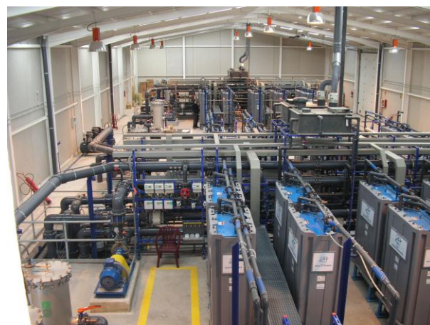
Figure 2: Installed EDR Systems
